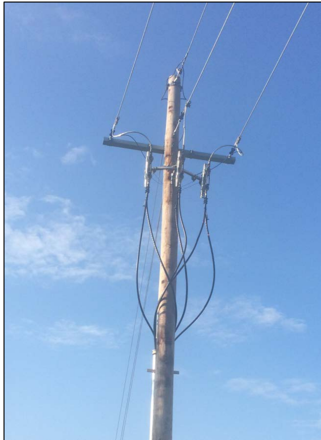
Figure 3.3 - Missing Arrestors on Riser Pole
