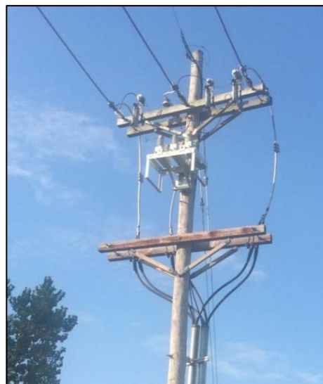
Figure 3.1 - Capacitor Bank Without Controls
