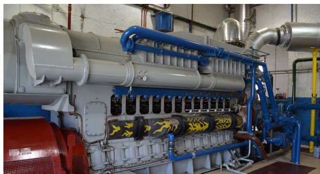
City of Wamego's Power Plant
